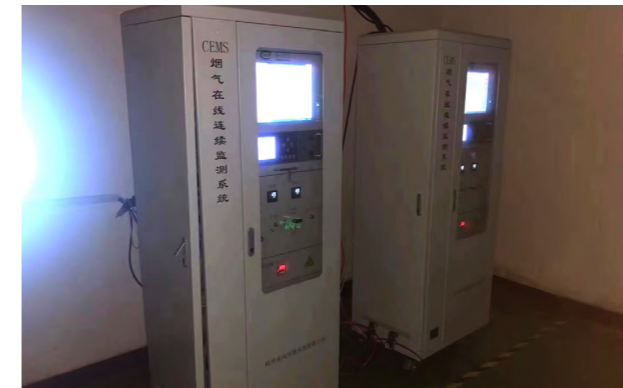
CEMS flue gas online monitoring system
