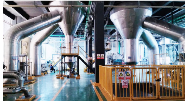
Central industrial base reused steam through sodium sulfate MVR evaporators
