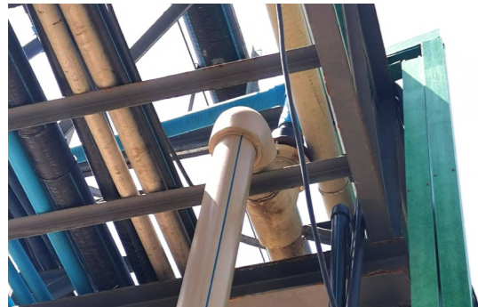
Western industrial base reduced the electricity consumption of raw liquor pumps by improving the feeding of raw materials
