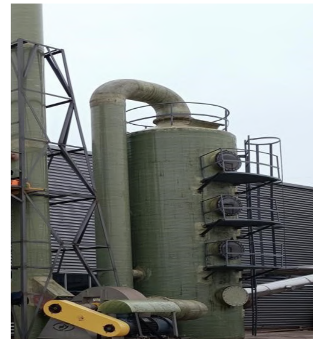
Water curtain-based dust removal tower
