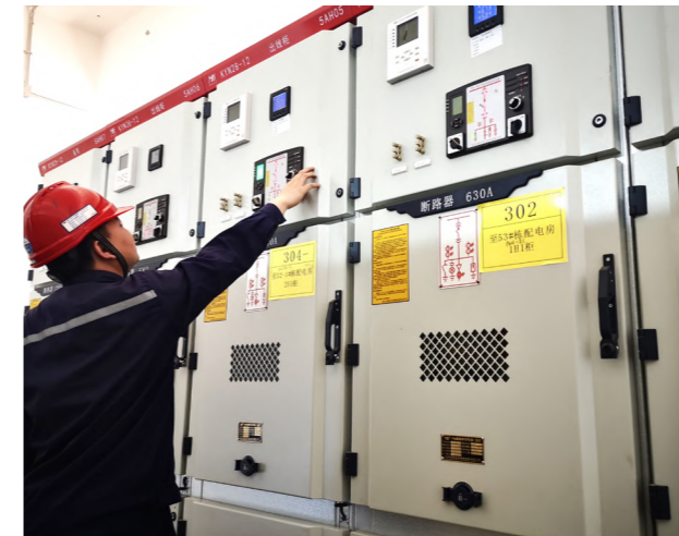
Meter readers regularly record energy consumption
