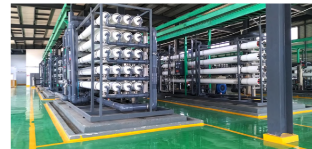
Reverse osmosis - pure water production workshop in central industrial base
